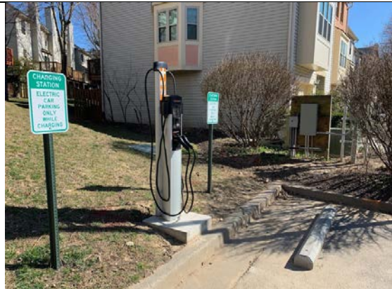
Another view of the station showing the other side of the electrical panel.
