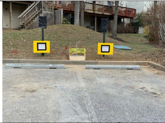
Temporary signage near the concrete pedestal. Note that the "EV only" signs are temporarily covered up.
