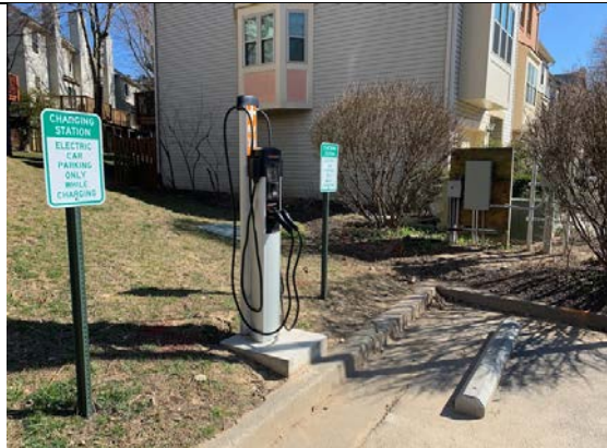
Another view of the station showing the other side of the electrical panel.
