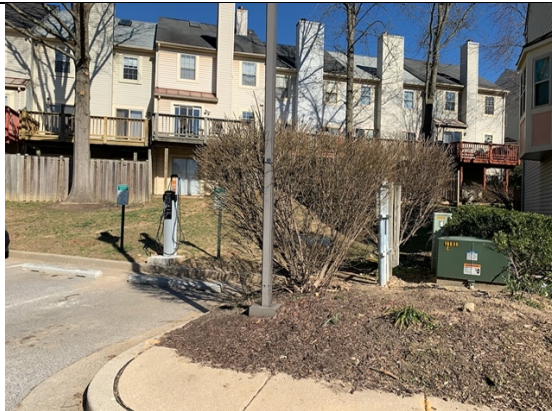
A view of the station showing the nearby transformer and electrical panel.
